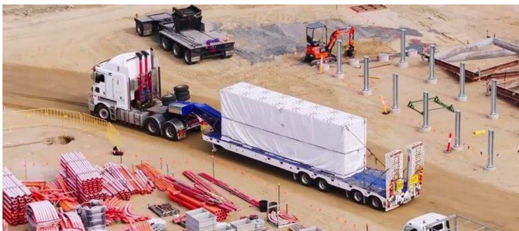
Figure 3-3: Battery Energy Storage Units shown on low loader combination
