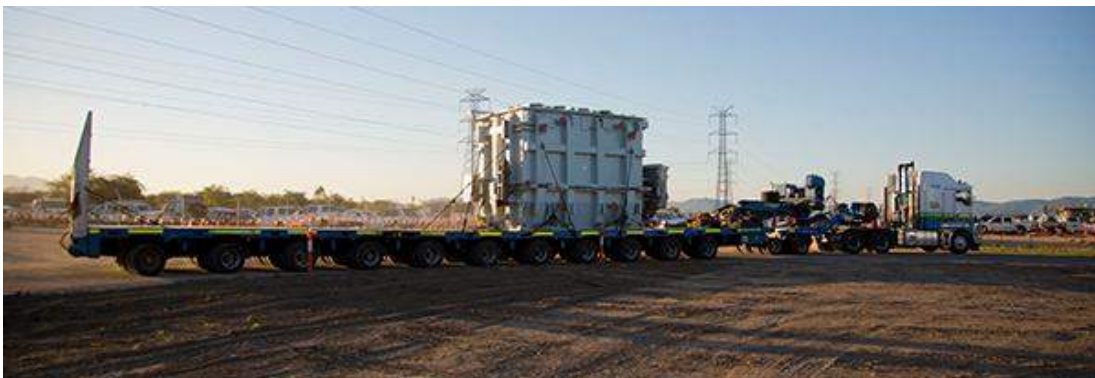
Figure 3-6: 132/33kV HV Transformer
