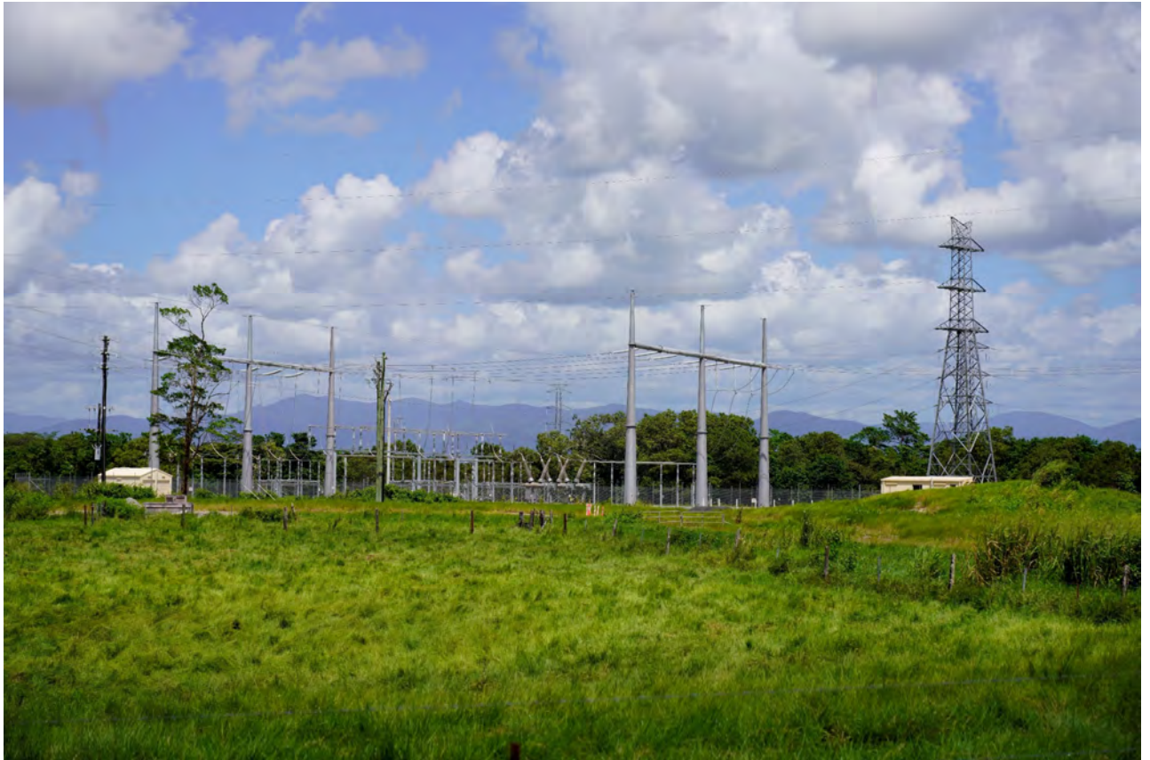
FIGURE 4-6 VIEW TO NEW TULLY SUBSTATION FROM TULLY GORGE ROAD
