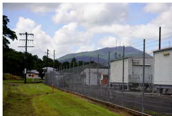
FIGURE 4-1 VIEW FROM SANDY CREEK ROAD TO POWERLINK TULLY SUBSTATION
