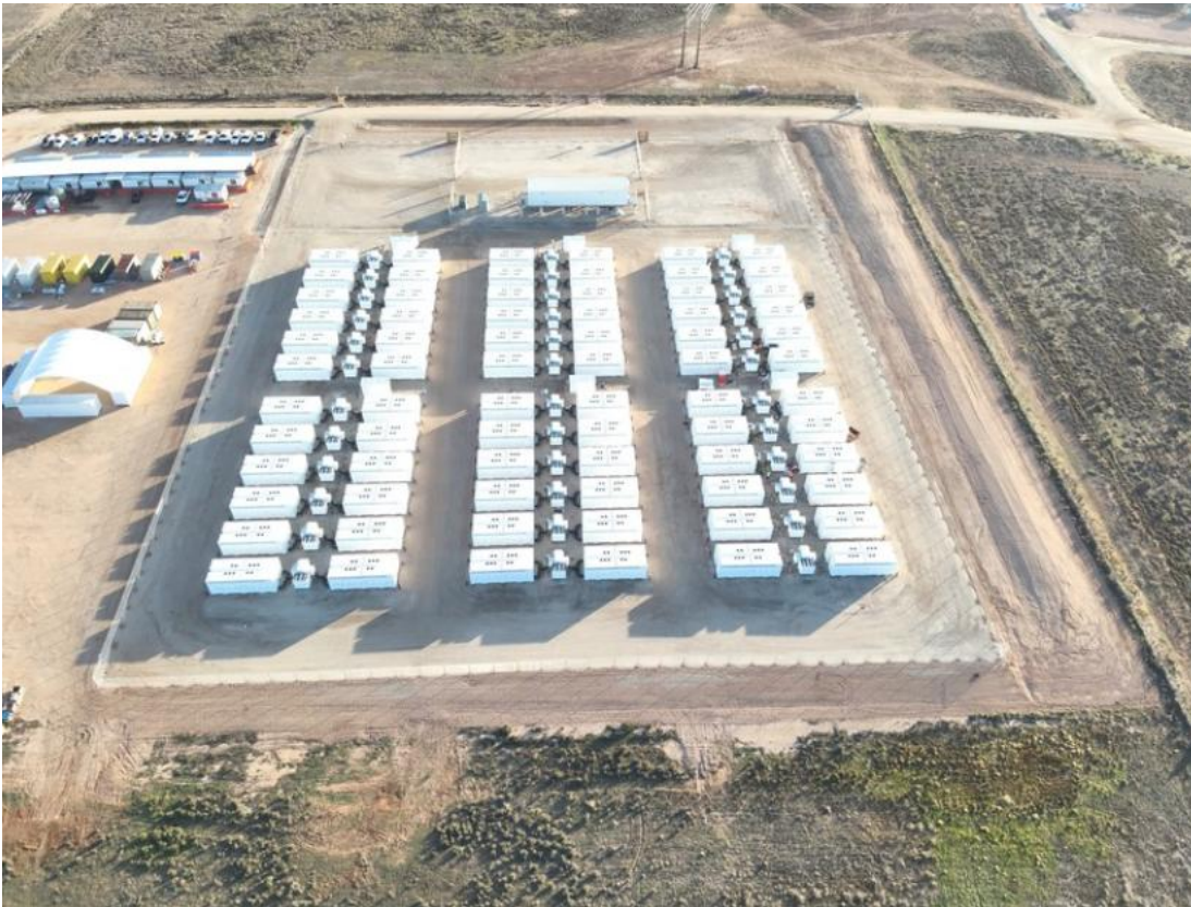
FIGURE 4-3 LIMONDALE BATTERY STORAGE UNIT
