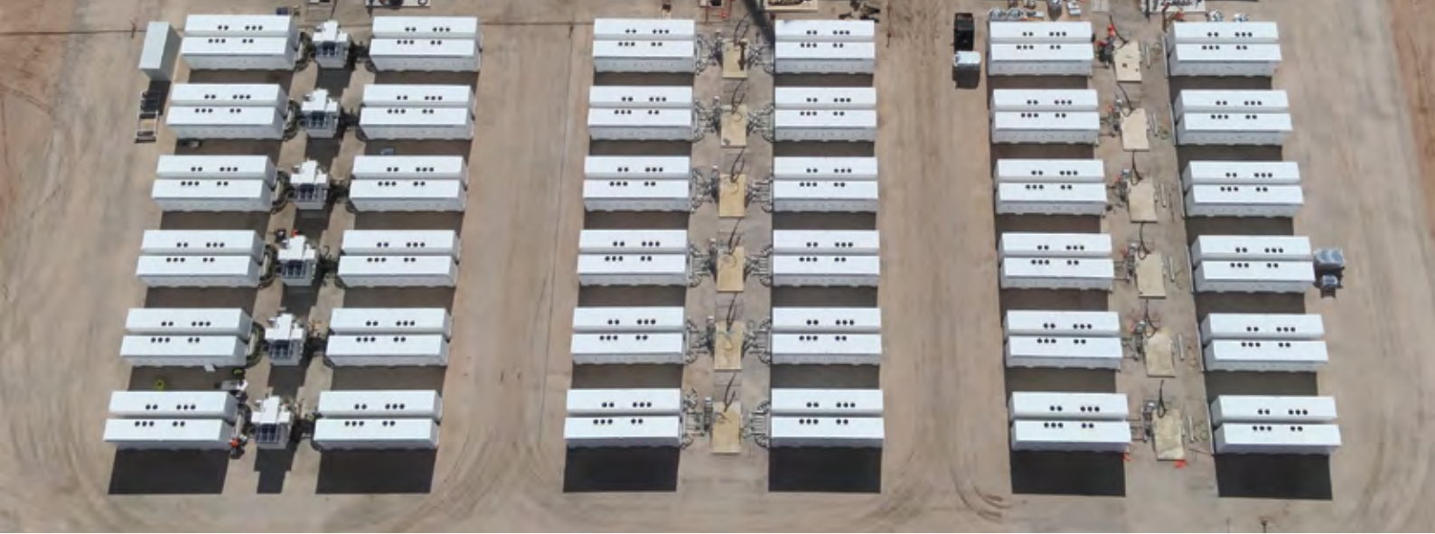
RWE's Limondale BESS, near Balranald in New South Wales.
