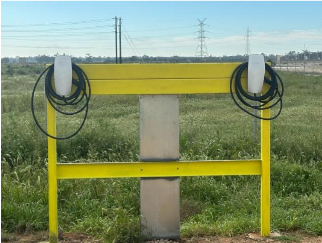
Electric Vehicle Charger
