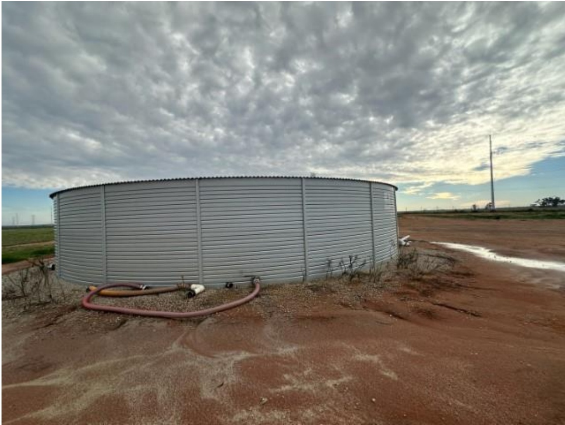
Fire Fighting Water tank
