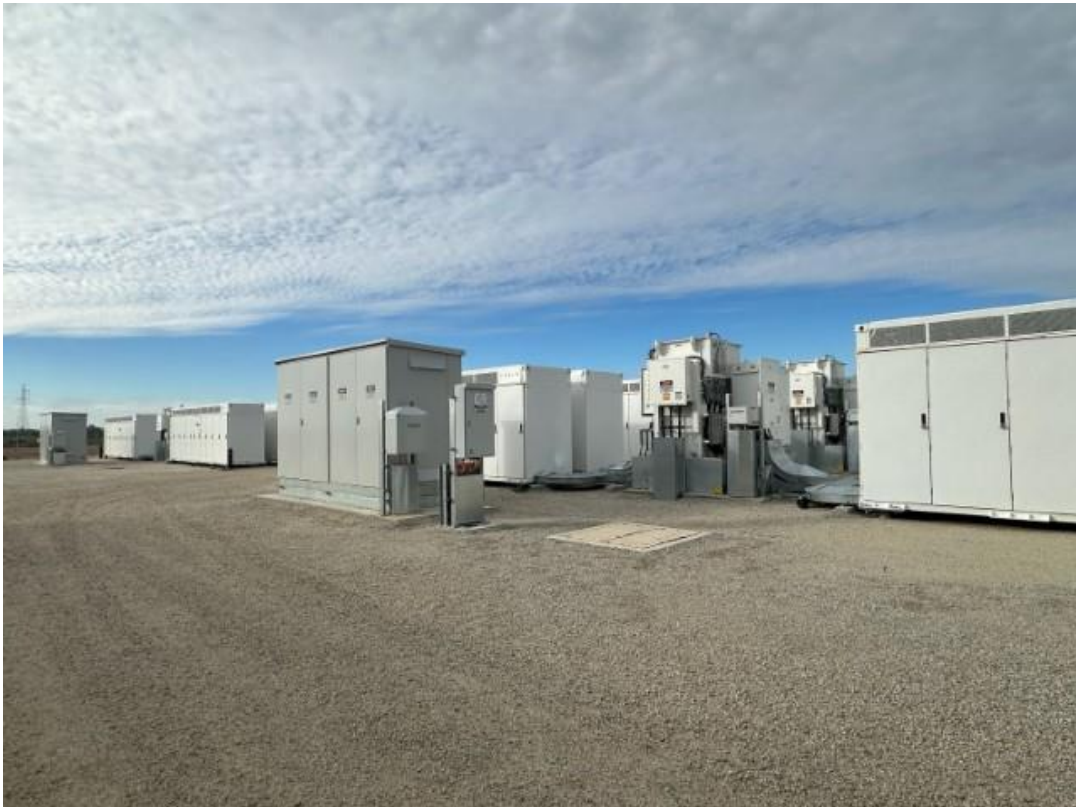
Battery Energy Storage System Components
