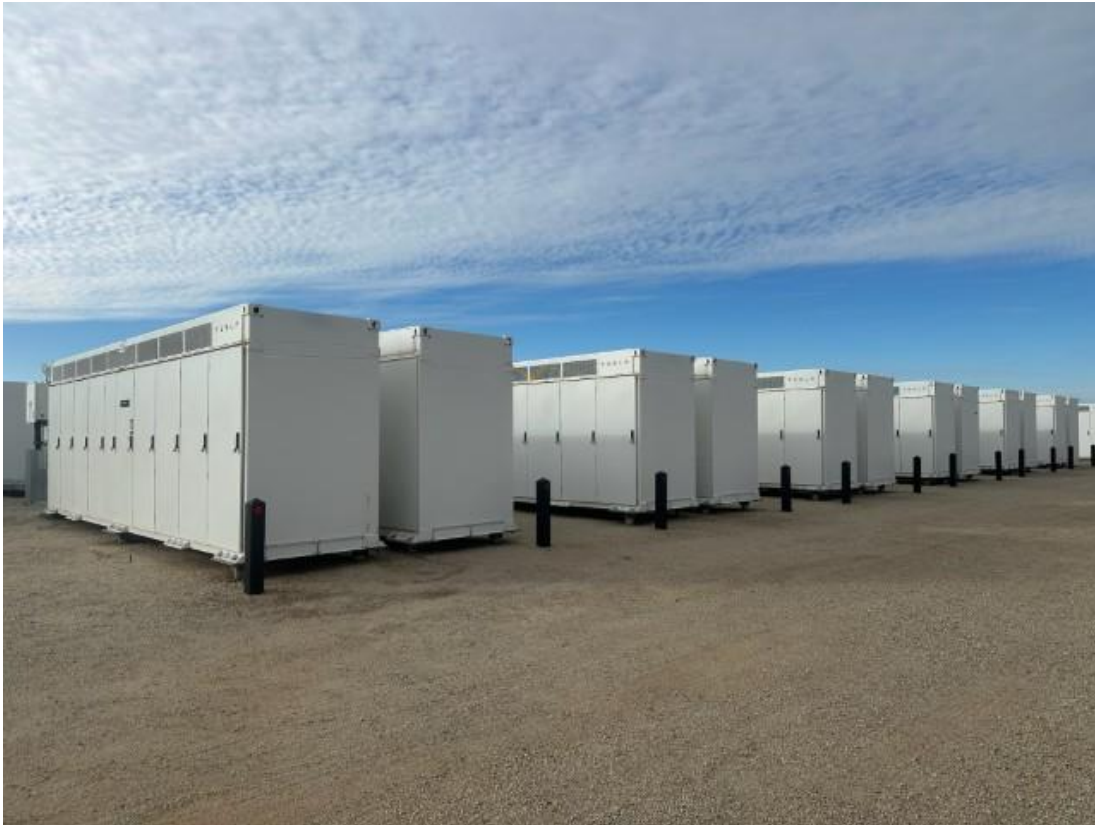
Battery Energy Storage System Components
